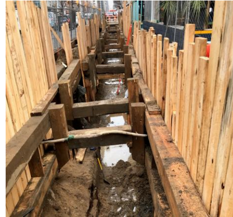
Preparing trench where the new 36" Trunk Water Main in the east side of 3 rd Ave between E 33 rd St and E 34 th St
