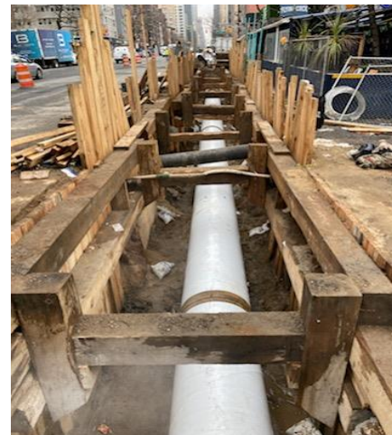
The installation of the new 36" Trunk Water Main pipe, in the trench (shown above), on the east side of 3rd Ave between E 33rd St and E 34th St
