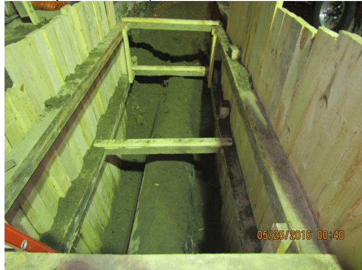
Removal of trunk water main on Park Ave W between E 42 nd St and E 41 st St
