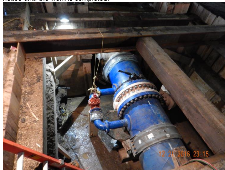
Installation of 36" trunk water main on E 42 nd St, west of Lexington Ave
