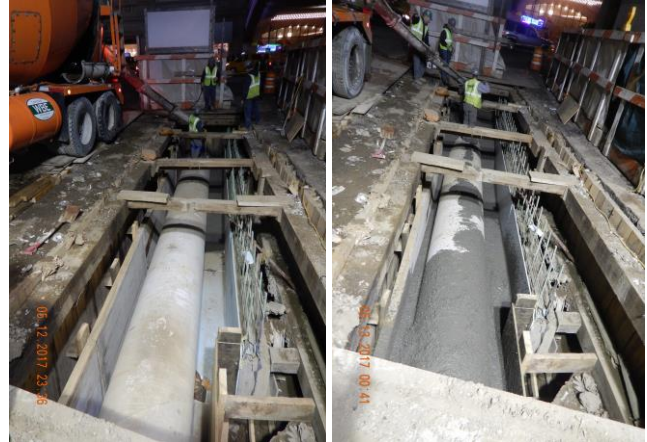
36" Trunk Water Main Concrete Encasement on Park Ave W. btwn E 42 & E 41 Sts.
