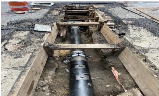
Newly installed Con Edison gas main along Park Ave. East from E. 40 th to E. 41 st Streets looking north.
