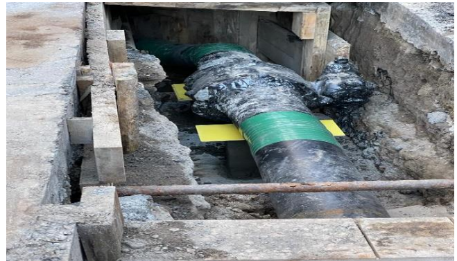
Newly installed Con Edison gas main valve along the intersection of Park Ave. East & E.41 st Street looking west.
