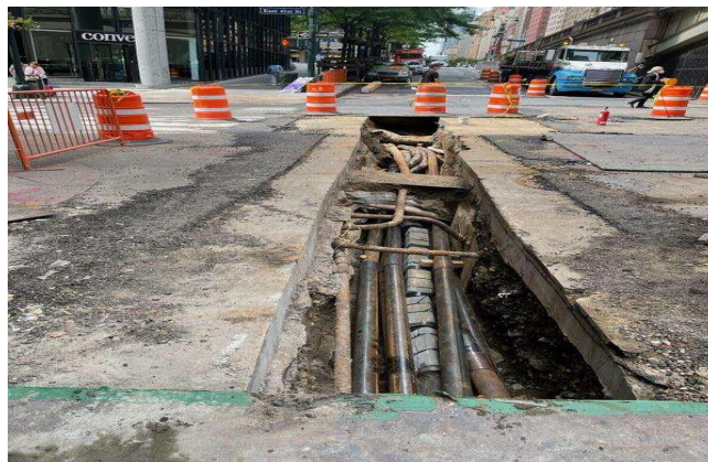
Installation of Con Edison Electrical Steel conduits along Park Ave. East between E.41 st and E.42 nd Streets looking South.
