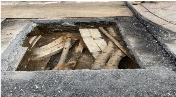
Exploratory utility test pit along the southeast quadrant of E.41 st St./Park Ave.
