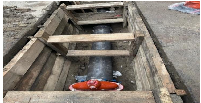
Newly Installed 12" water main along Park Ave East between E. 41 st to E. 42 nd Streets looking north.
