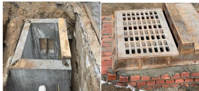
Installation of a catch basin along the Southeast Corner of Park Ave. East between E. 41 st and E. 40 th Streets.
