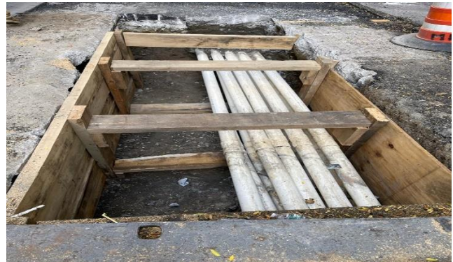
Preparations for the ECS facilities relocations along Park Ave East between E. 40 th to E. 41 st Streets looking north.
