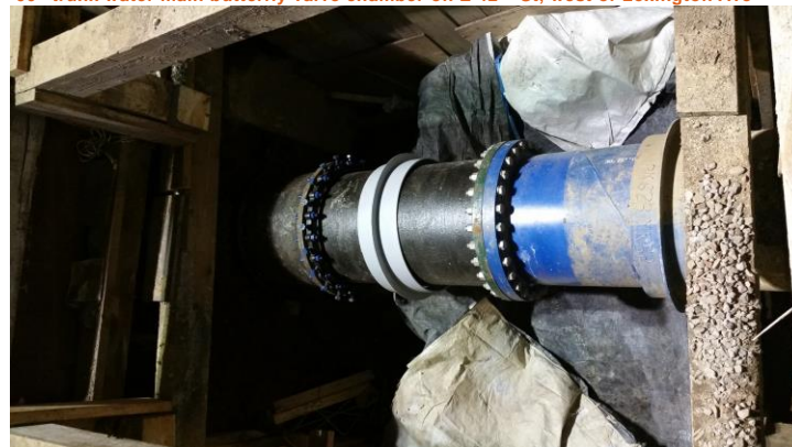
Installation of 30" trunk water main insulated joint on E 42 nd St, west of Lexington Ave
