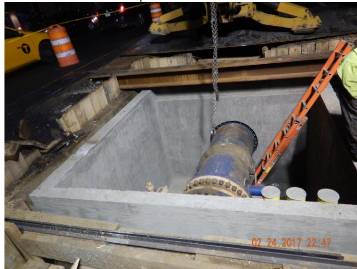
36" trunk water main butterfly valve chamber on E 42 nd St, west of Lexington Ave
