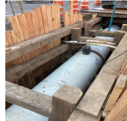
48" steel Trunk Water Main pipe on the west side of 2nd Ave. between E. 32nd St. and E. 34th St.
