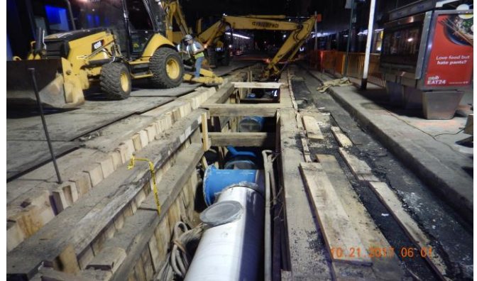
Installation of 36" trunk water main on E 40 th St btwn Park & Madison Aves.
