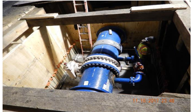
36" butterfly valve & chamber on E 40 th St btwn Park & Madison Aves.
