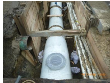
Trunk Water Main Installation on the west side of 2 nd Ave. between E. 35 th St. and E. 36 th St.
