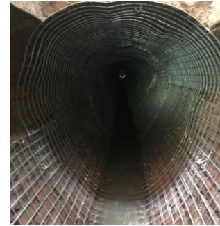
Sewer work on E. 35 th St. between 2 nd Ave. and QMT Exit
