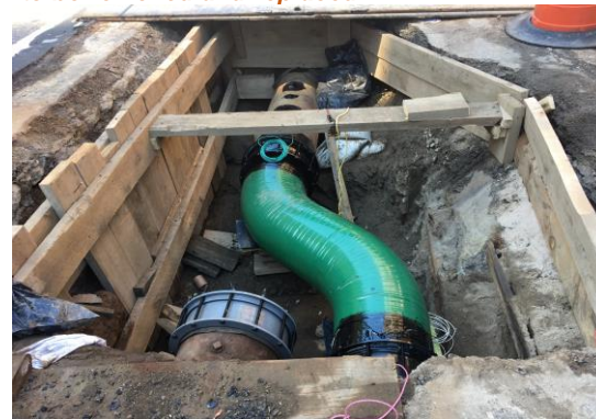
New gas main tie in to existing gas main at 3 rd Ave. and E. 33 rd St.
