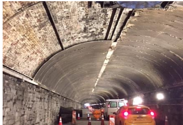
Corrugated metal ceiling panels are removed from the tunnel roof during asbestos abatement.
