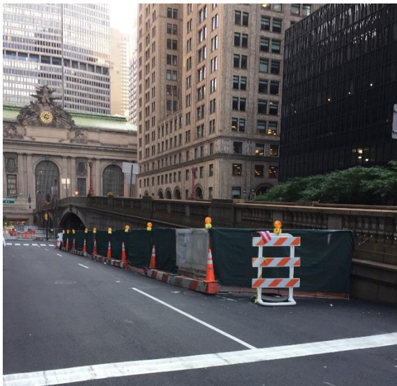
Green mesh netting covers the construction materials storage yard on Park Avenue at 40 th Street.
