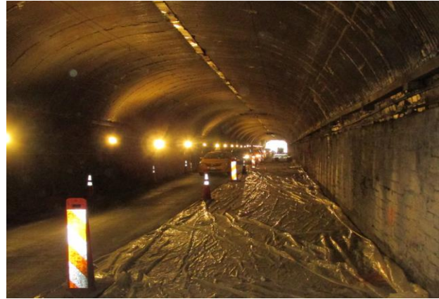
West side of the tunnel is prepared for installation of new roadway.
