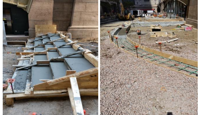
Plaza Work: concrete footing for granite stair treads (l) and river bench (r)
